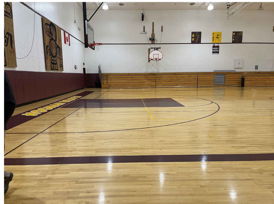
PHOTO 4: VIEW LOOKING WEST AT DEPRESSION
